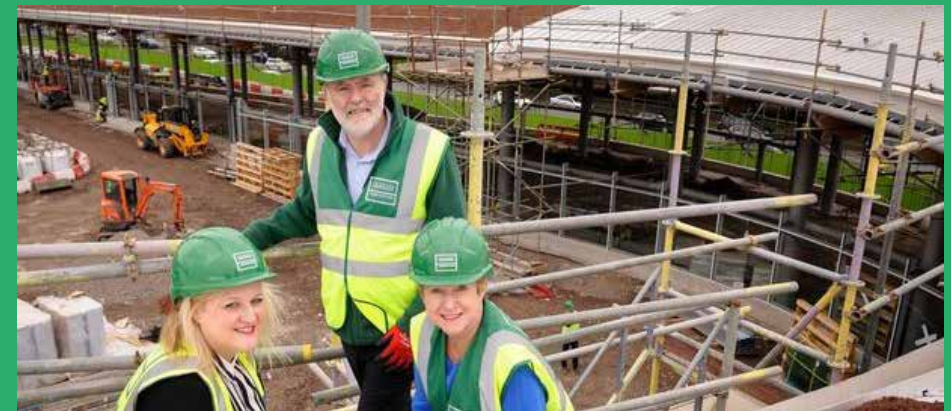
Christine with Cllr Karen Shore and Martin Bambrick, Graham Construction on the rooftop of the new Chester Bus Exchange
